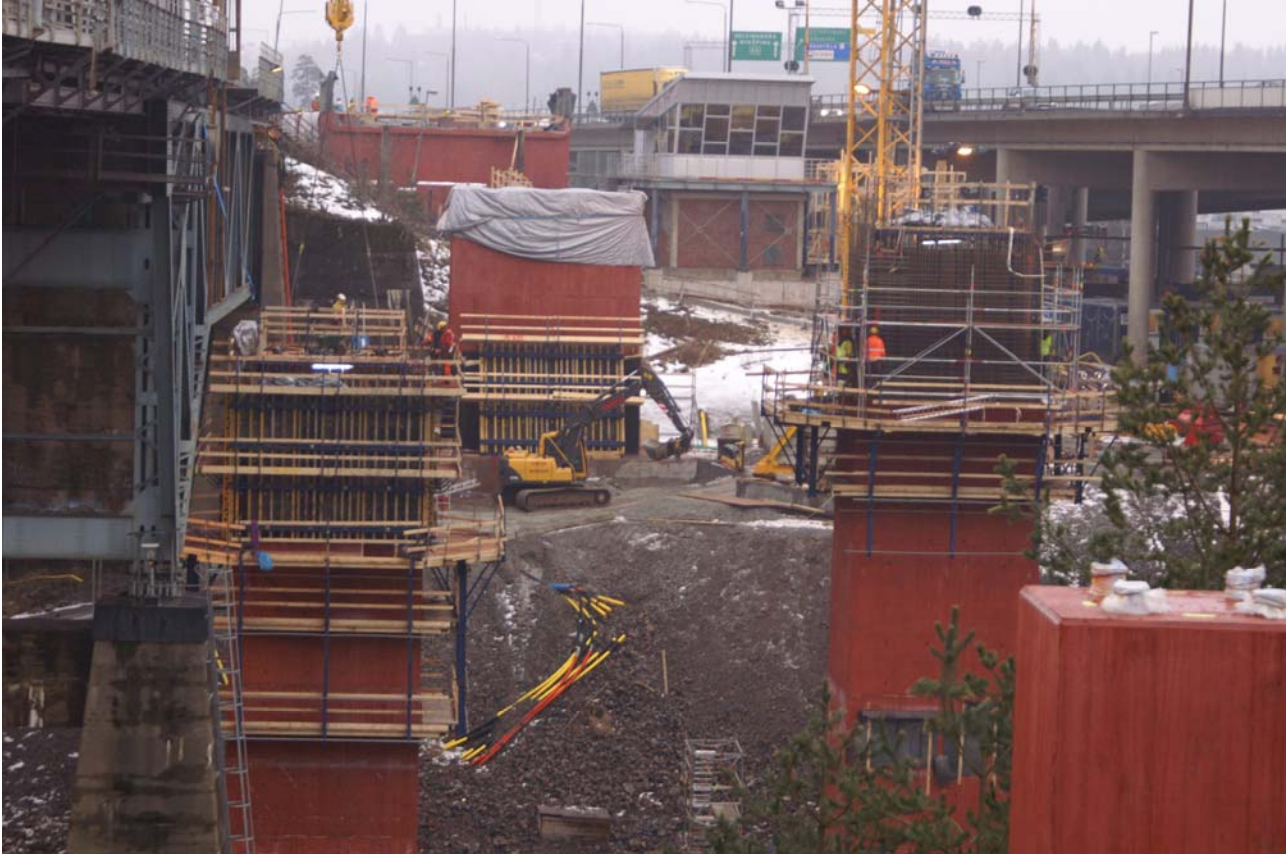
Figure 5. Structures with red concrete
